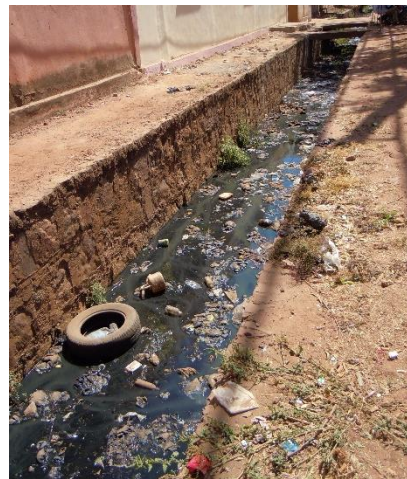
B: Stagnant Open Sewer
