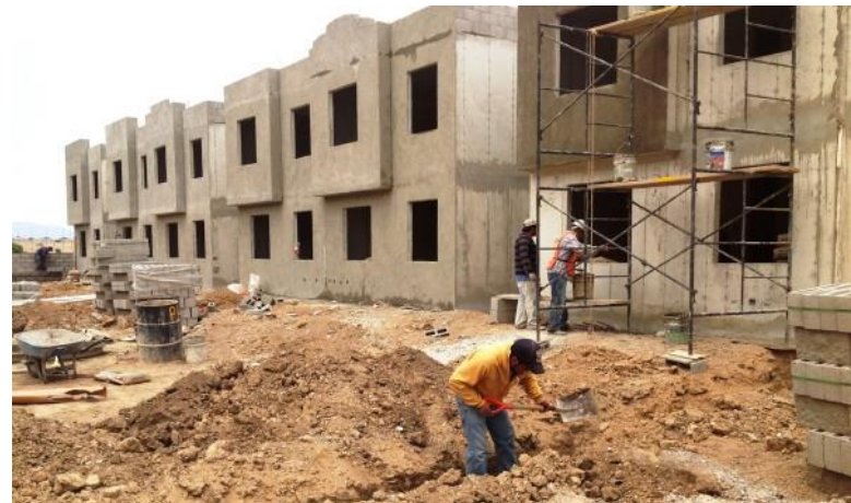
Workers from a Mexican construction firm build energy-efficient homes in Tula, in Hidalgo state. THOMSON REUTERS FOUNDATION/Monica Healy
