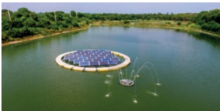
Figure 2: Floating SPV in Dhanas Lake, Chandigarh (picture provided by case study authors)
